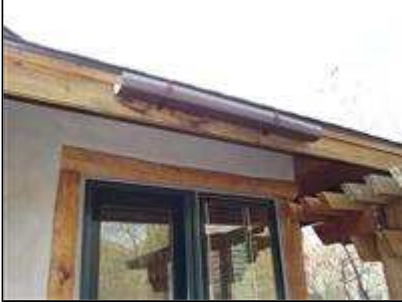
2.5 Picture 1 Gutter without downspout at north entry
